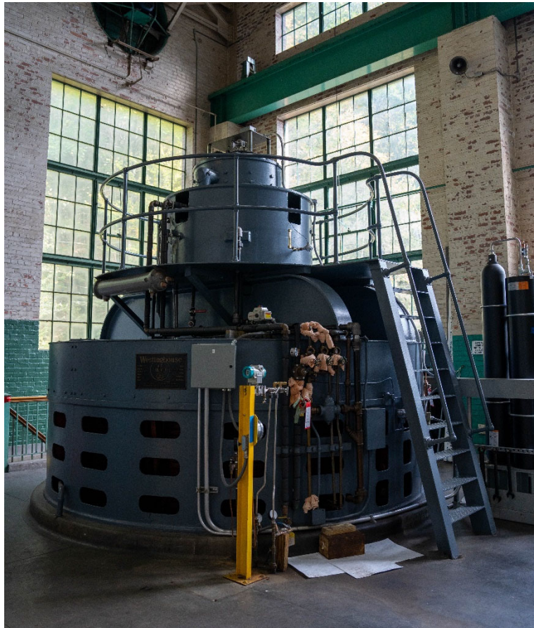
CMHS Existing Turbine #1
