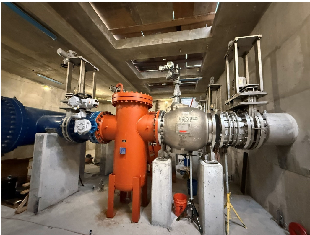
Energy dissipating valve assembly (AECOM photo, 12/08/2025)
