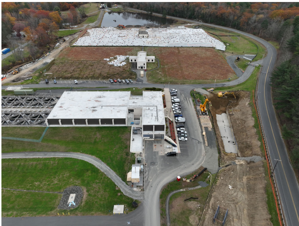
Excavation for 60-inch and 72-inch steel raw water piping (SWSC drone photo 11/05/2025)
