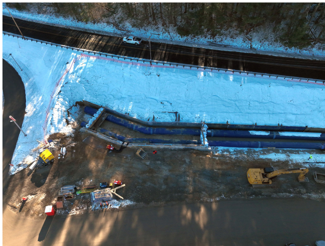
Construction of 60-inch and 72-inch steel raw water piping (SWSC drone photo 12/01/2025)
