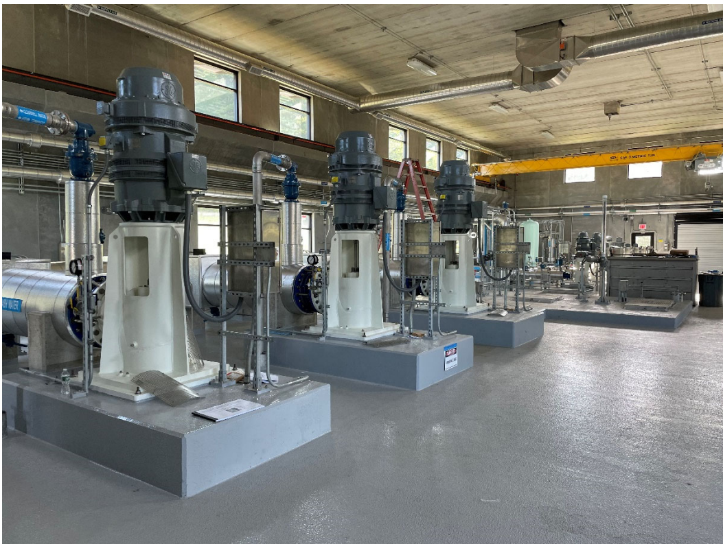
Backwash Pumps inside Pump Station, 09/26/23
