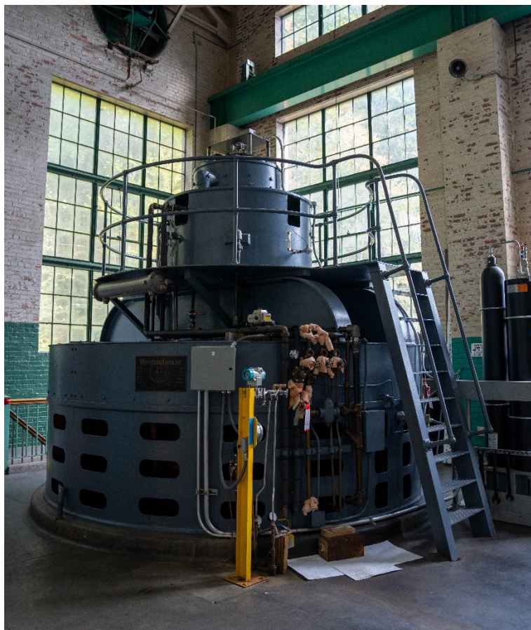
CMHS Existing Turbine #1
