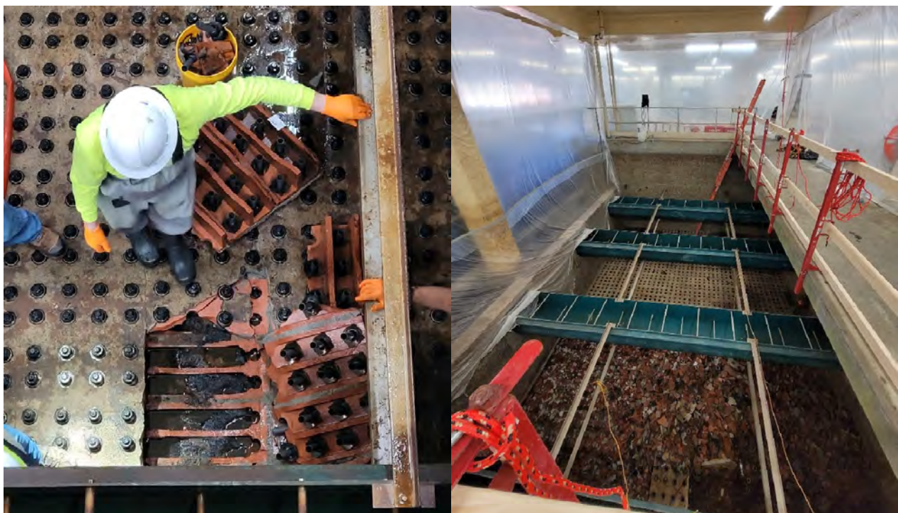
Left: failure of the filter underdrain. Right: demolition of the underdrain prior to installation of new system.
