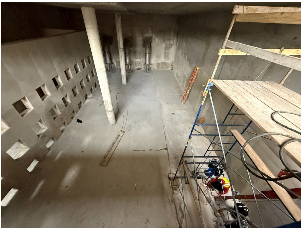
Equalization Tank interior (Engineer photo, 03/19/2025)
