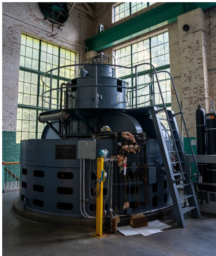
CMHS Existing Turbine #1
