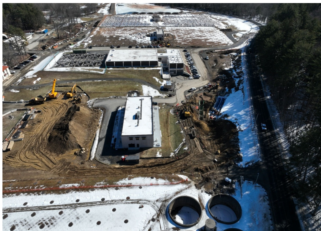
Construction of 60-inch and 72-inch steel raw water piping (SWSC drone photo 03/10/2026)
