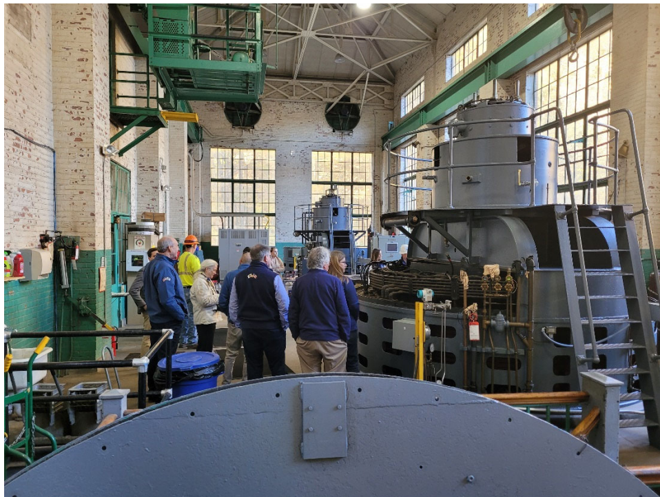
Inside Cobble Mountain Hydroelectric Station during a visit from Congressman Richard Neal in October
