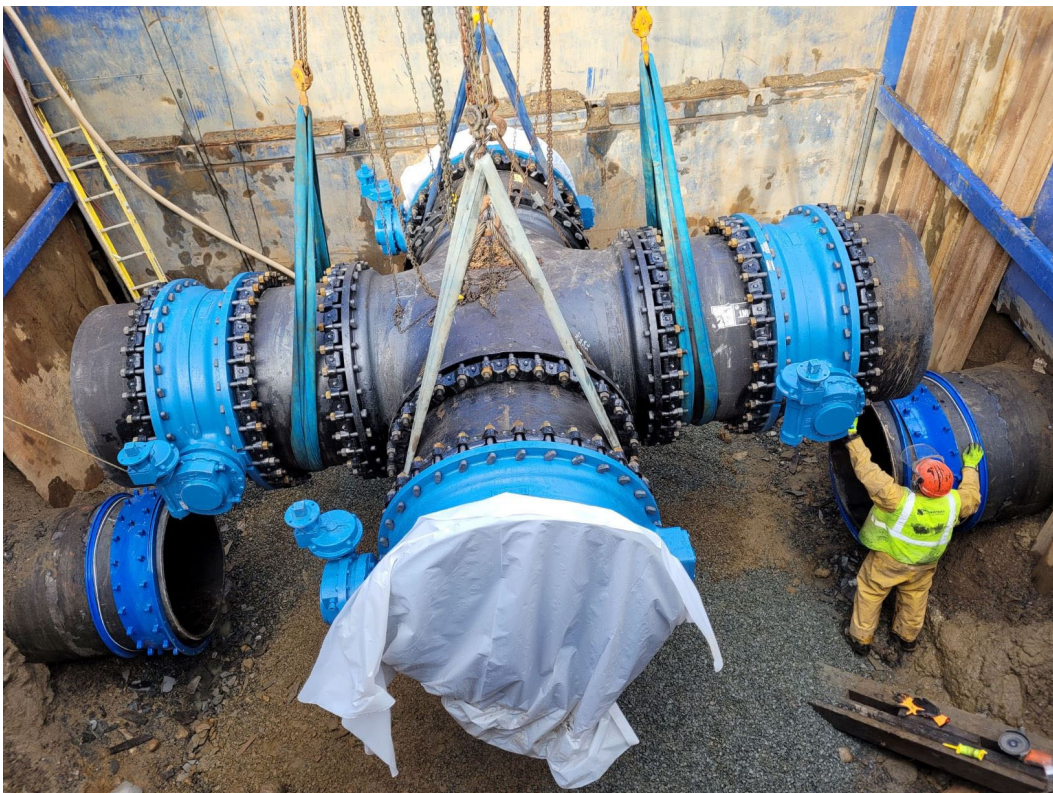
Installing 48-inch ductile iron cross into existing 48-inch steel rapid sand filter effluent pipe
