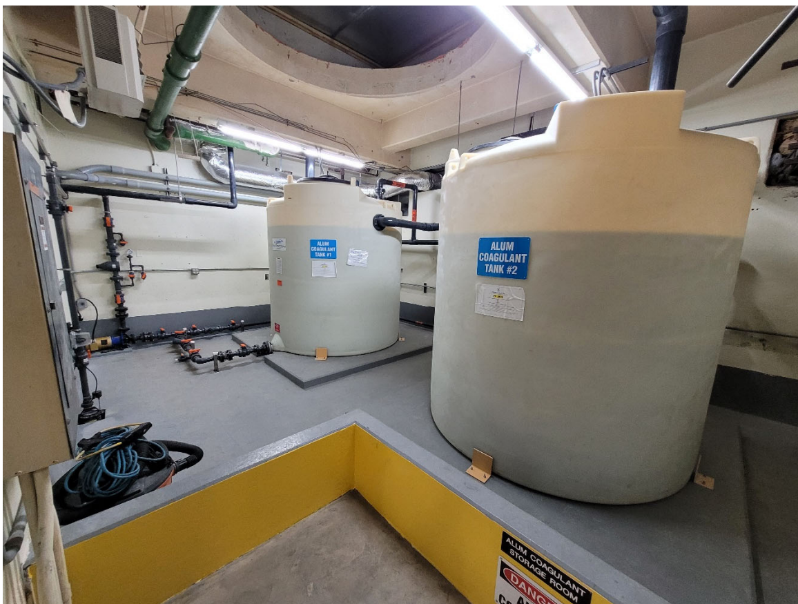
New bulk storage pads and secondary containment in the new ACH storage room.
