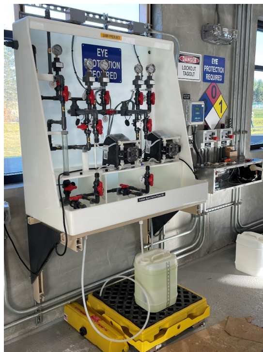
Domestic Water Sodium Hypochlorite Booster System
